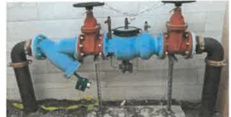
Backflow Preventor Photo
