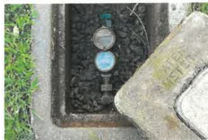
Water Meter Photograph-New
